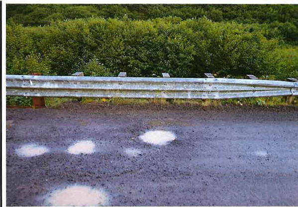
Bridge No. 2213 Br. Name Barney Creek Date 09/25/24 Inspector Jones / Landes Frame 18 Near End Upstream Transition Rail File P9251568.jpg
