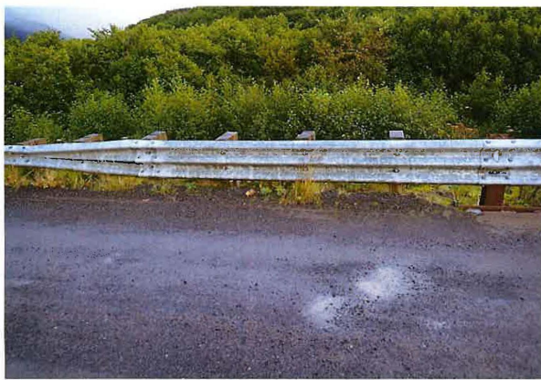
Bridge No. 2213 Br. Name Barney Creek Date 09/25/24 Inspector Jones / Landes Frame 17 Far End Upstream Transition Rail File P9251583.jpg
