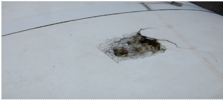
Typical isolated areas of insulation damage
