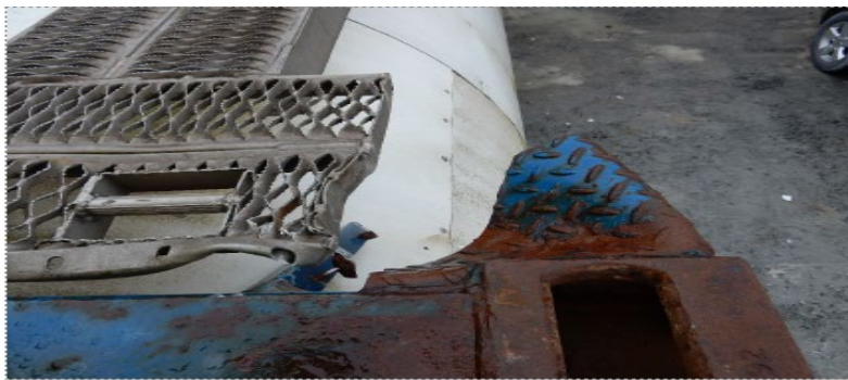
Steel support structure and adjacent steel walkway were observed to be deformed on the upper Northwest corner
