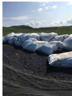
Nelson Lagoon Erosion Project
