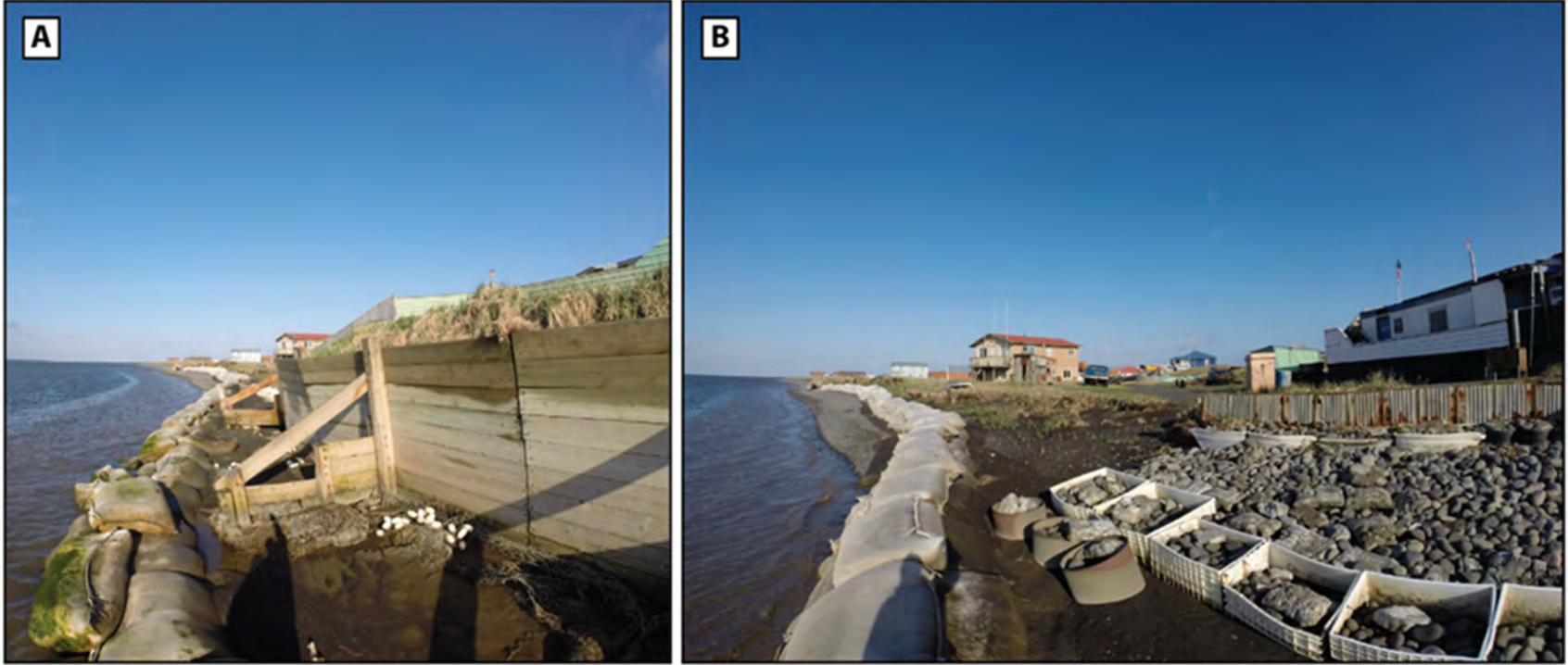
Figure 27. Seawall and sediment containers in place along the lagoon coastline of Nelson Lagoon. May 2019, UAF-ACGL.
